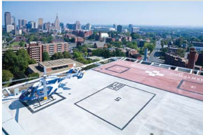
Petra recently completed renovations to the helipad on the roof of Hartford Hospital.
